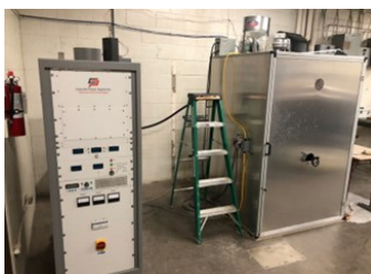
The complete RF system, including generator (left) and the vertical applicator with the container door closed (right).
