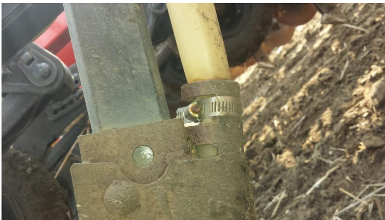
Figure 15. Collapsed hose due to an overtight hose clamp.
